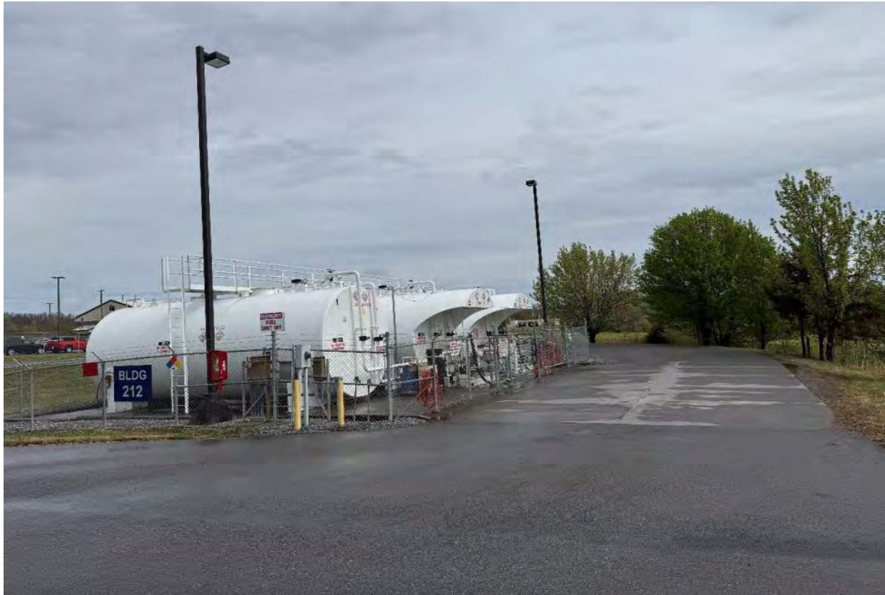
17 Tri-Cities Airport Fueling Facility - Facing N.jpeg
